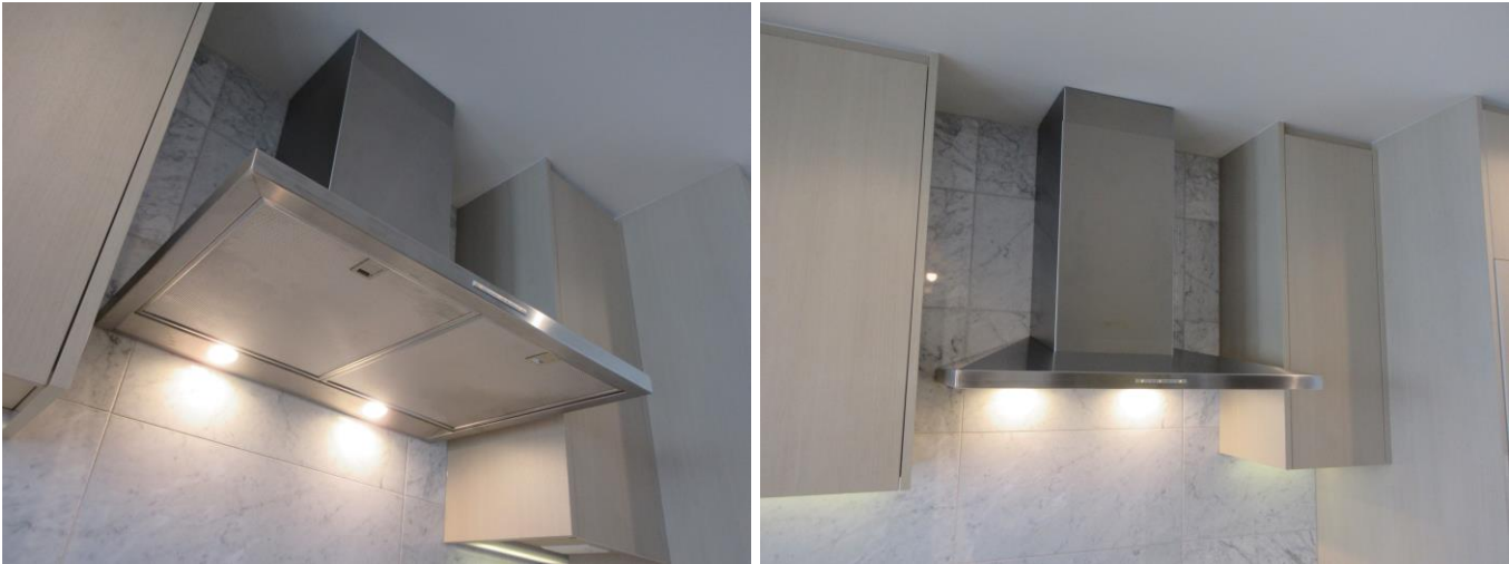
The house had electrical range hood. The range hood electrical exhaust fan was tested and was functional at the time of this home inspection.
