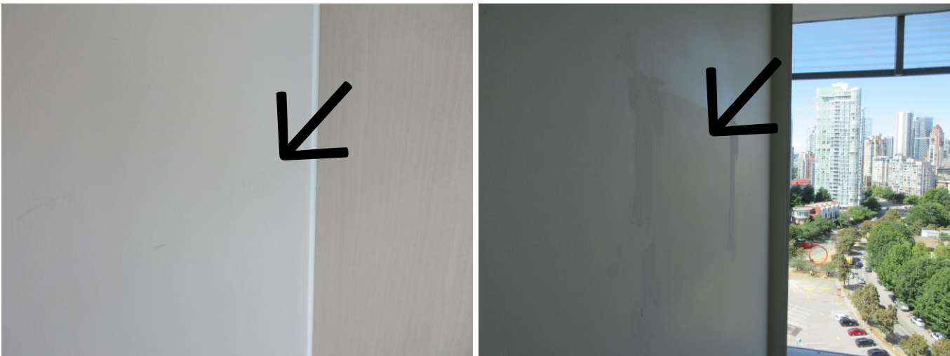
The wall paint was damaged, and missed, on the living room wall. It is likely to be cosmetic issue. I recommend re-painting the wall.
